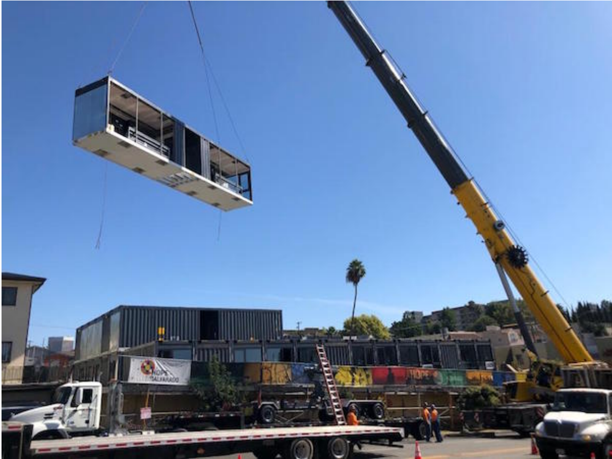
A crane lifts a module onto the Hope on Alvarado project / Photo: KTG Y Architecture + Planning
